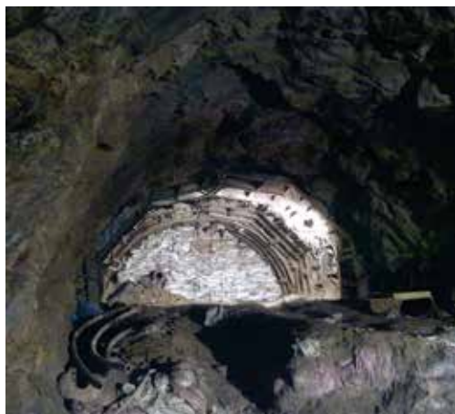
Picture 1 Photograph of HRT- Face 2 at ch.1170 m taken during site inspection
