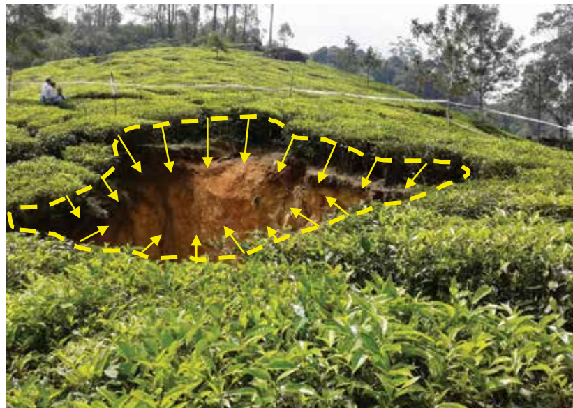
Picture 2 Surface depression at ch.1170.50 along HRT – Face II alignment
